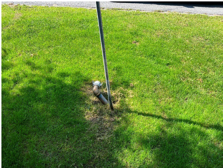
BLOWOFF – WOODSIDE DRIVE
