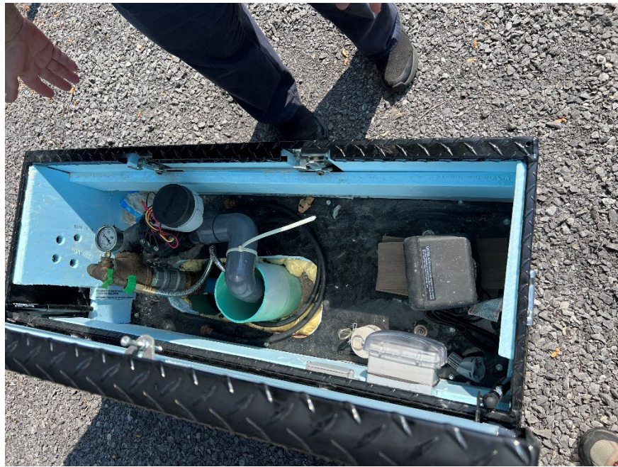
FLUSHING HYDRANT OFF IVES STREET
