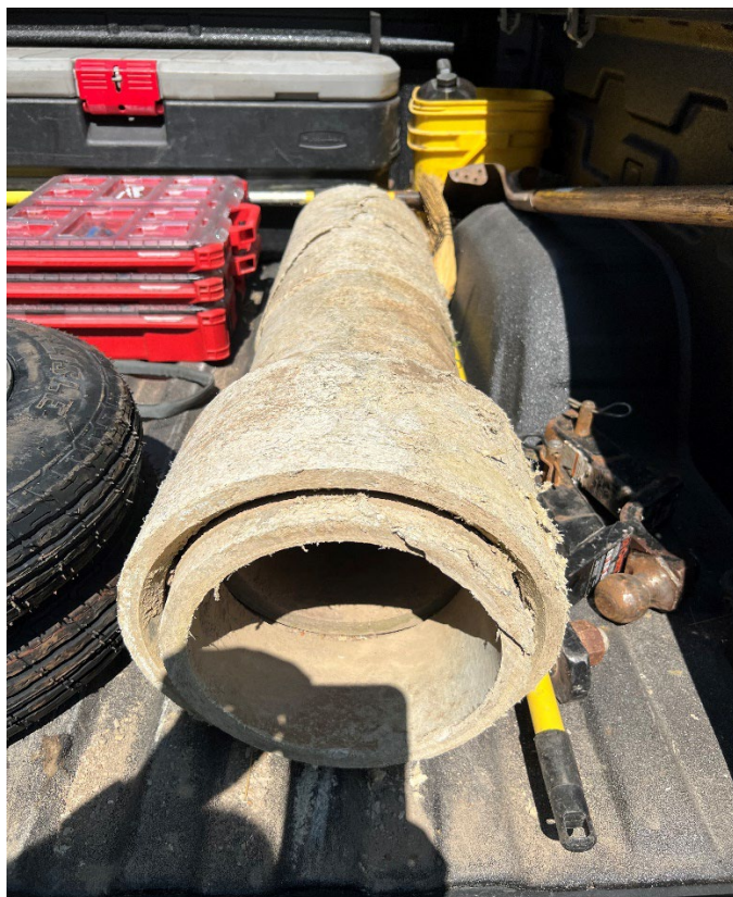
SECTION OF WATER PIPE – LONGITUDINAL CRACK
