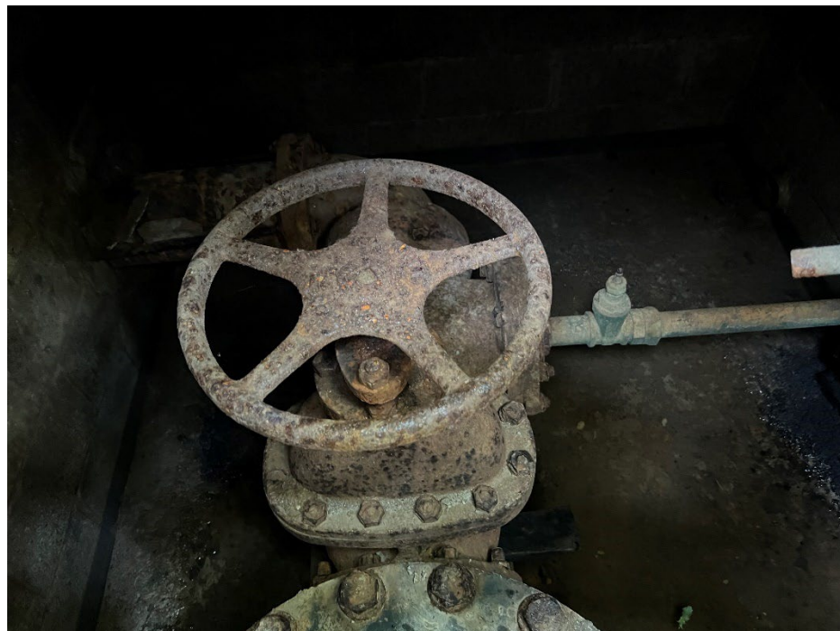
WATER MAIN VALVE IN METER PIT
