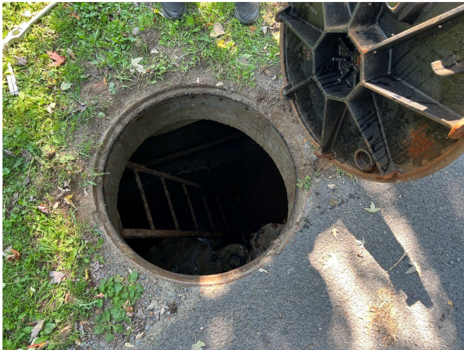
METER PIT – HOLCOMB STREET
