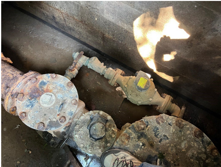
PIPES AND VALVES IN METER PIT
