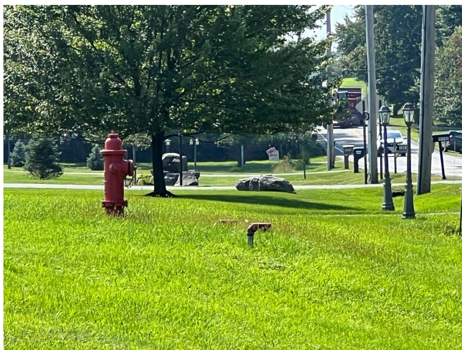
HYDRANT AND BLOW OFF
